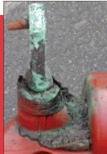
A typical fault
