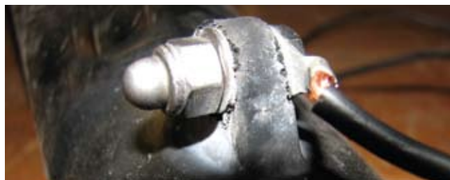
View of a termination with visible PD
