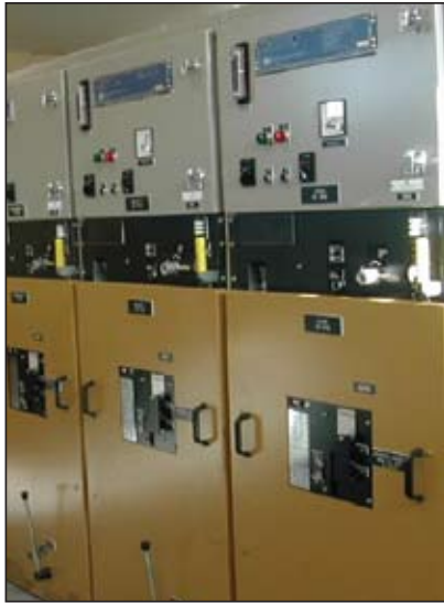
View of Fluair 400 Indoor Switchgear. It looks normal but a fatal failure is in progress.
