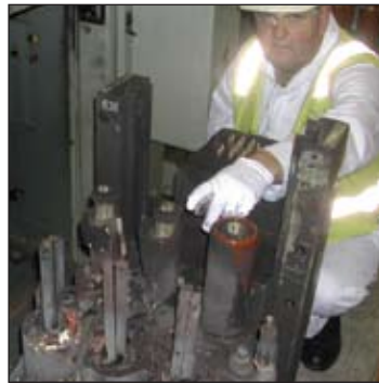
Failed AEI circuit breaker
