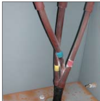
Termination failure in process (21-2-08)
