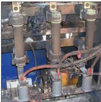
Generator Termination failure in process (21-1-08)
