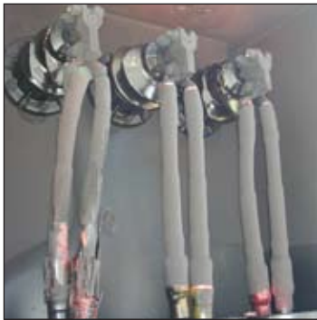
Termination failure in process (21-12-07)
