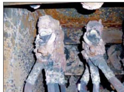
Figure 3 Remains of failed termination (Original cause of failure)
