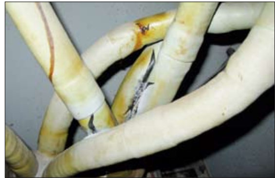
Figure 1 Failed termination located by Partial Discharge Engineers. Failing to locate this in a timely manner would have resulted in Figures 2 & 3 occurring.
