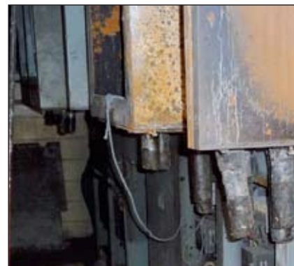
Figure 2 Termination failure, lead to entire HV switchboard failure (The rust is caused by foam used by the fire brigade)
