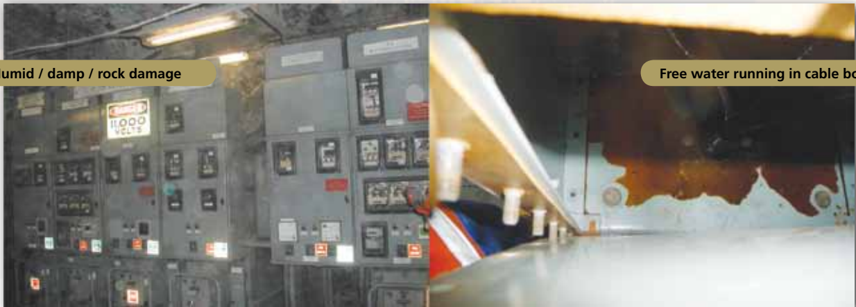
An example of the environment that a Mining substation has to operate in.
