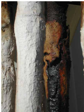
An example of what was found once the cable was dug up.
