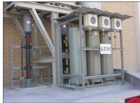
View of a typical SF 6 cable termination.
