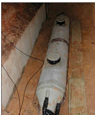
View of an exposed stop-joint prior to On-Line Partial Discharge survey.
